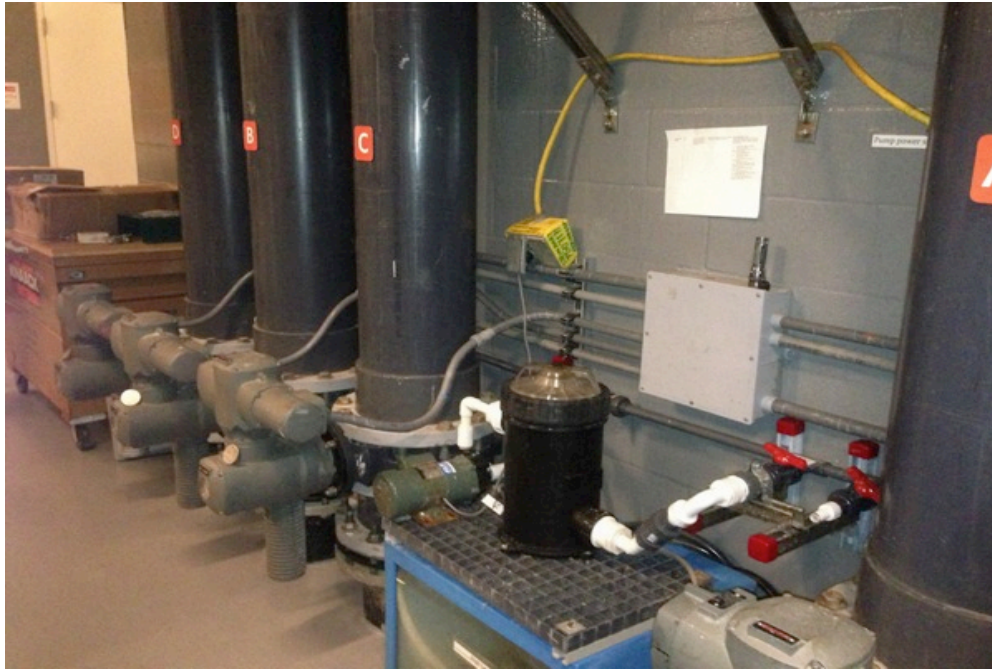
Photo 3 : The zone injection feeding system between the closed loop zones waiting for final plumbing and electrical work. Photo R. Ross
